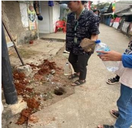
Figure 1. The process of digging the soil with a depth of 10 - 30 cm to make biopore holes
