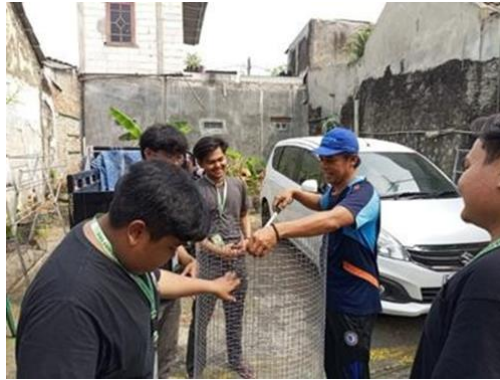
Figure 5. Measure the length of the RAM Wire, then cut the wire, with a circular position made linked to a fellow wire that has been made into a circular position from concrete.
