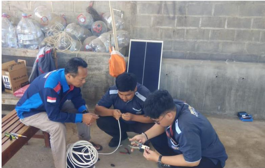
Figure 6. Solar panel wiring and connection assembly
