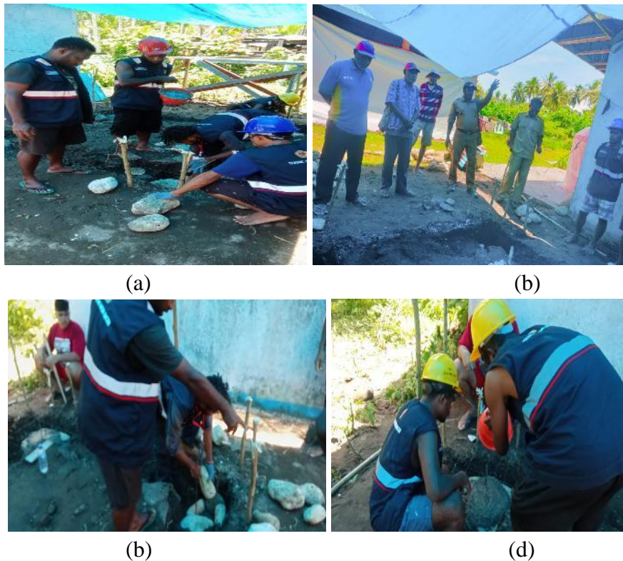
Figure 3. Initial activity stages: (a) Installation of foundation stakes, (b) Excavation of foundations, (c) Installation of foundations, and (d) Casting of foundation corners.
