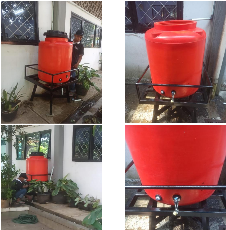
Figure 8. Torn collecting AC wastewater
