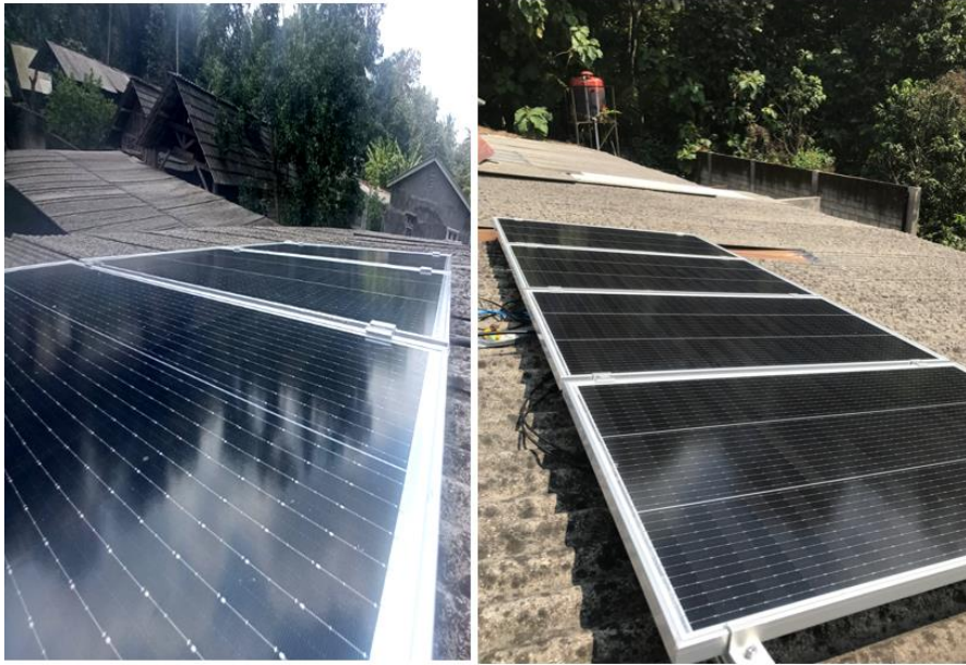
Fig.6 The results of installing solar panels in an open area
