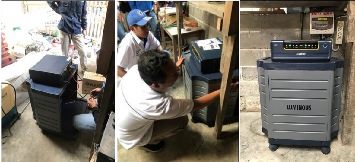
Fig.7 Smart inverter and battery installation in plastic box
