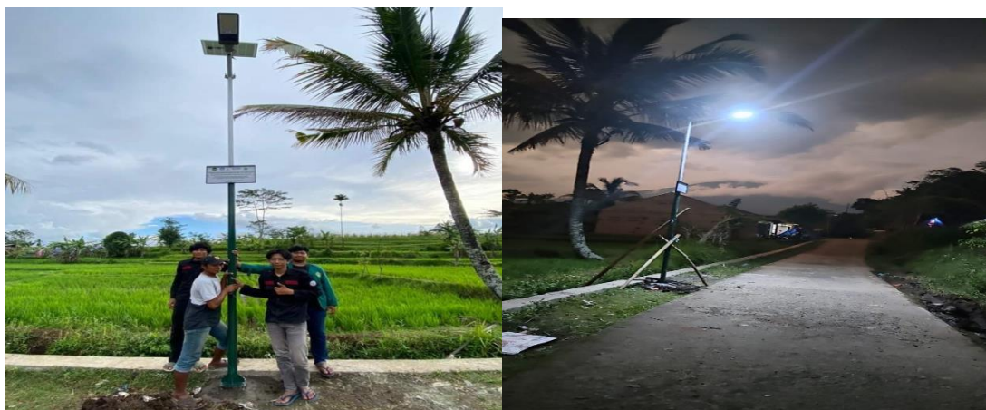
Figure 8 shows the PJU Solar Cell lights that have been installed and illuminate the surrounding area.
