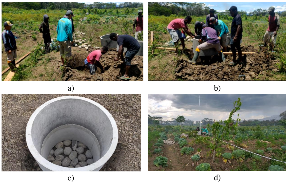
Figure 3: Overview of the Assistance Process for Making Joint Wells; figure a) the process of digging the points of multiple wells, b) The process of moving Bis into the dug hole, c) a picture of one of the several wells that are ready to be cast and d) the pipe installation process
