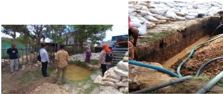
Figure 4. (above) Checking the location of construction infrastructure, and (below) Purchase of materials and lining for settling tanks prior to construction
