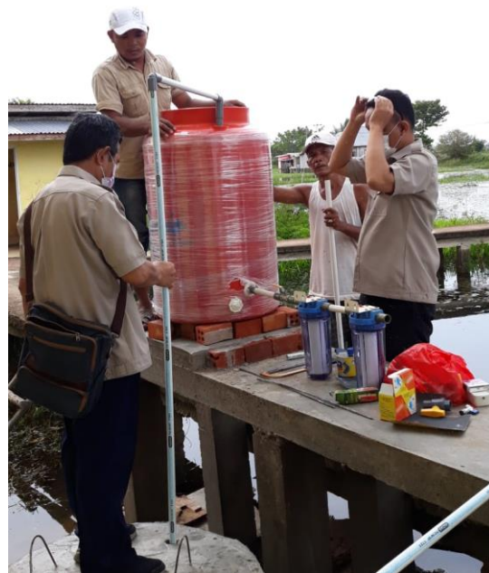
Figure 2. The process of making storage media and water treatment for dug wells Source: Community Service Activity Report
