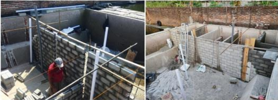
Figure 7. The process of installing bricks for the manufacture of pond filter tanks
