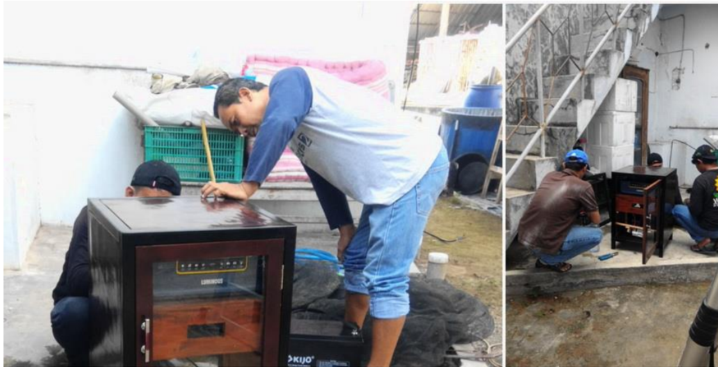
Figure 10. The process of setting the smart inverter and battery on the panel box
